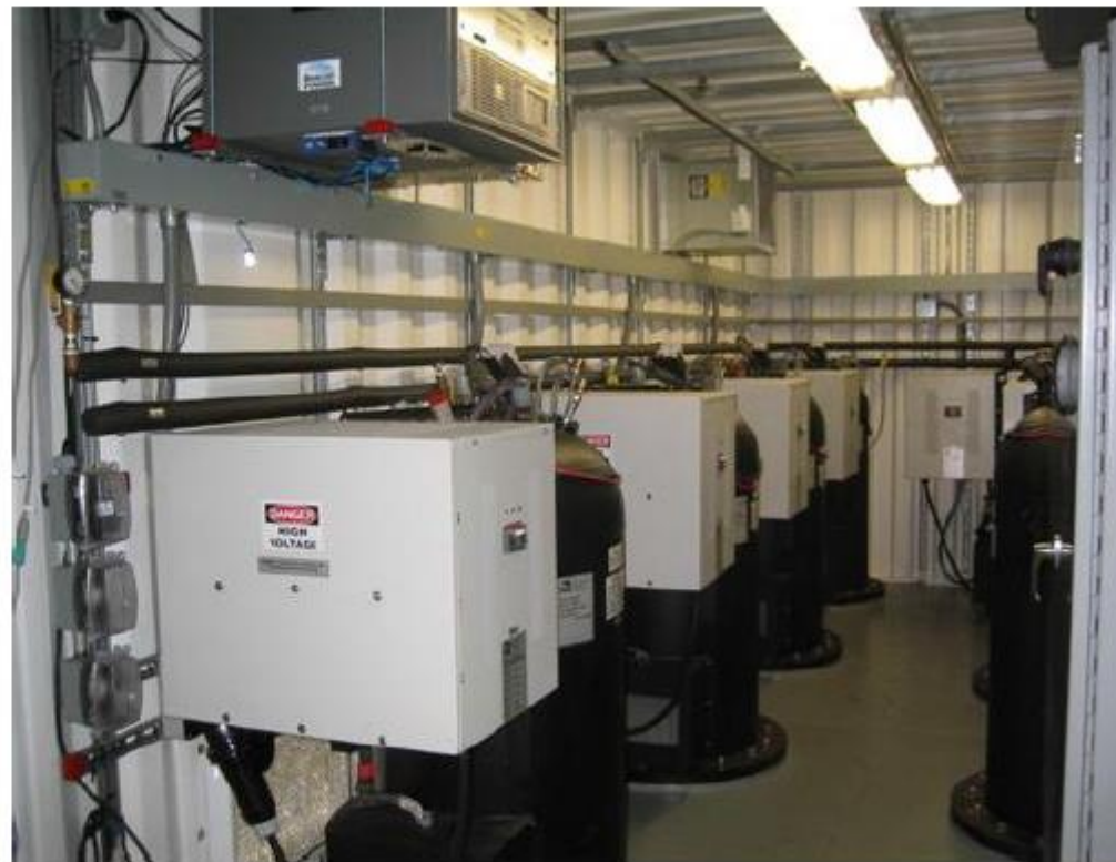
Beacon Power Corporation
