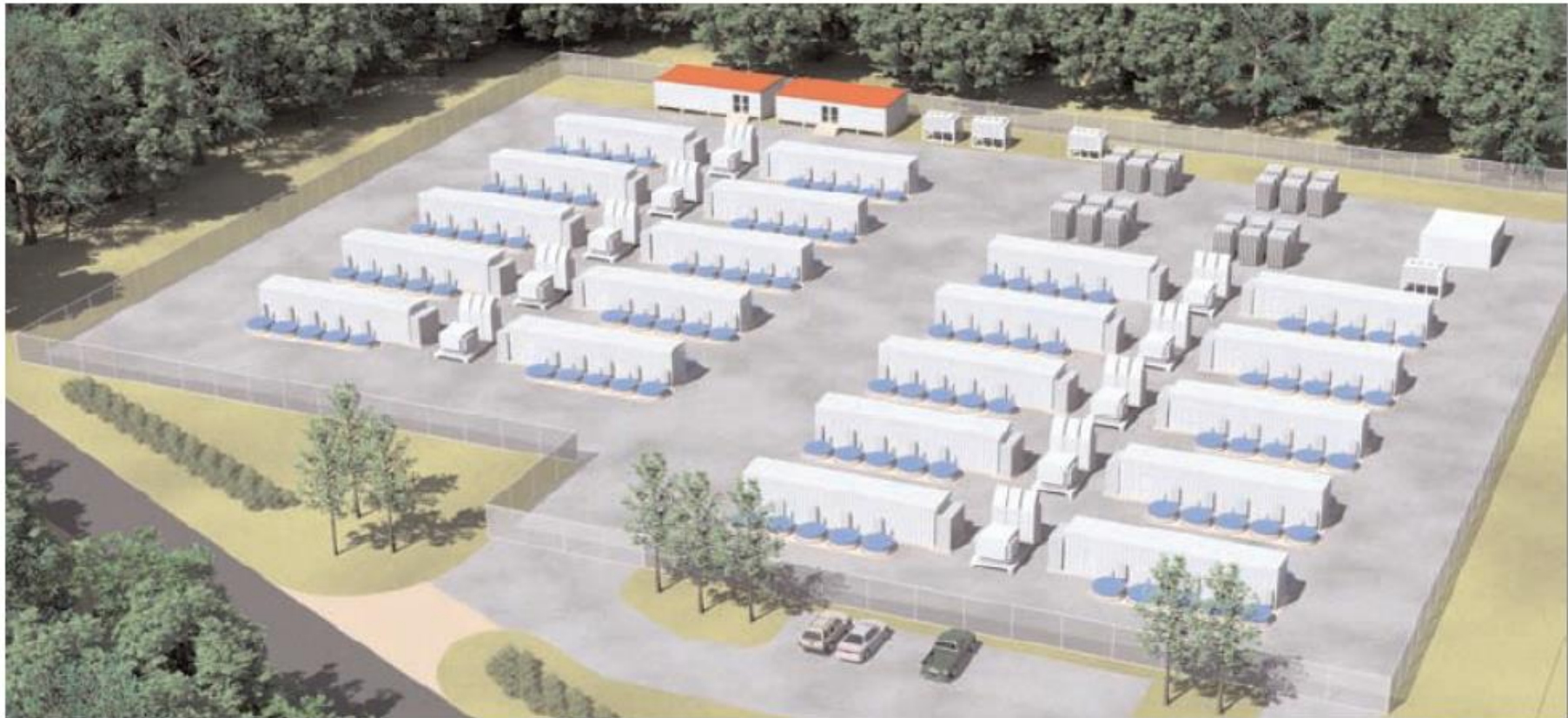
20 MW frequency regulation (Stephentown, NY, USA) July 2011
